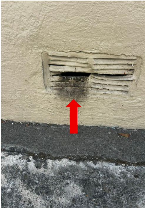
A damaged vent screen with evidence of rub marks from rodents.
